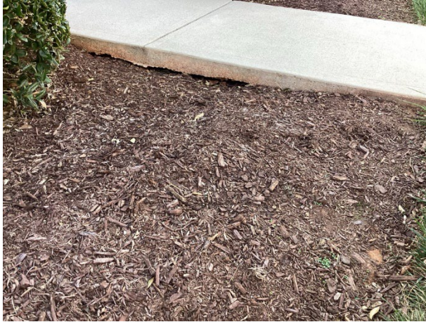
Soil undermining at sidewalk
