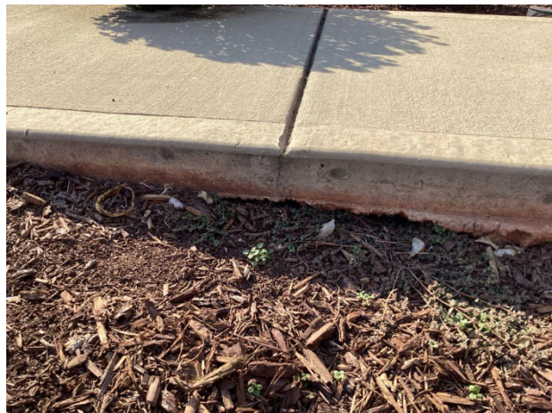
Soil undermining at sidewalk
