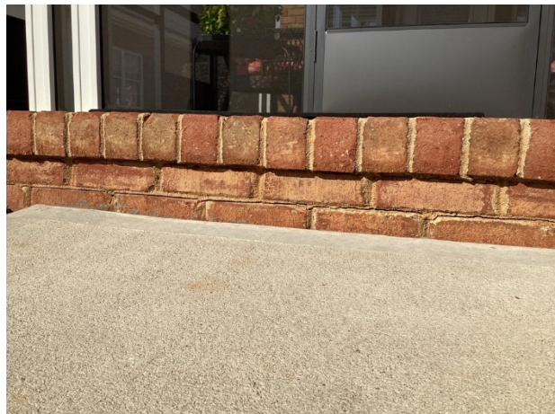
Masonry cracks beneath patio
