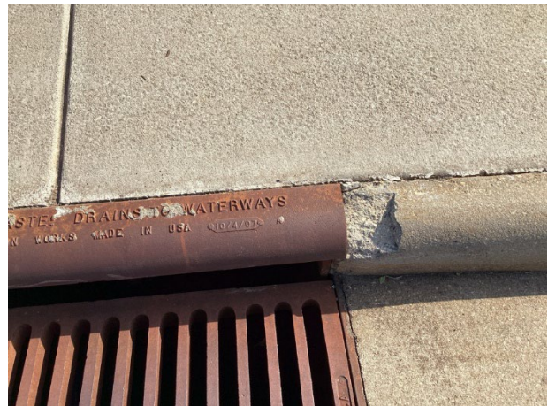
Catch basin collar damage
