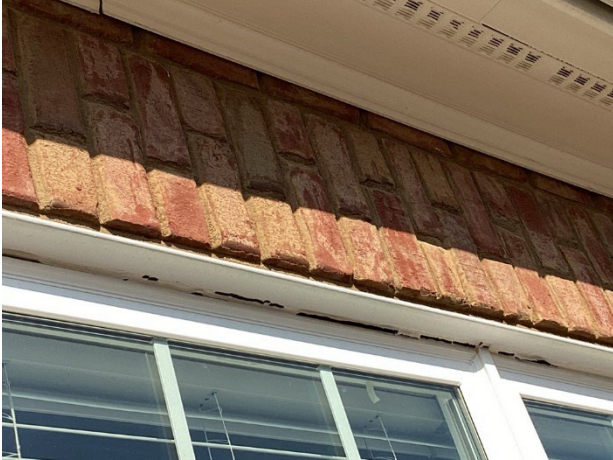
Sealant deterioration at steel lintel
