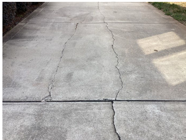
Driveway settlement near unit 8622
