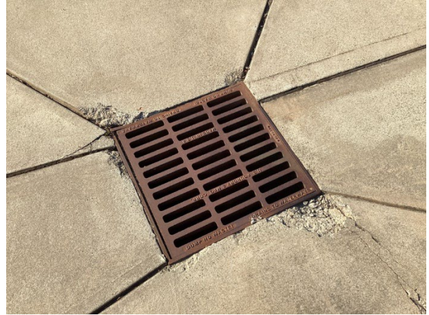
Spalling at catch basin
