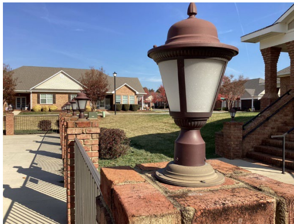
Exterior light fixture
